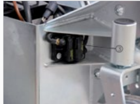
Abb. 76: Main safety switch
