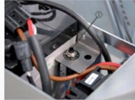
Abb. 77: Sec. safety switch, activ.
