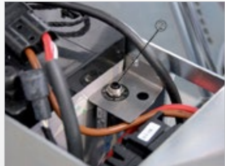
Fig. 116: Secondary safety switch
