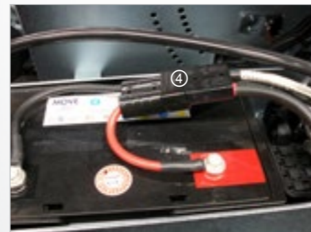
Fig. 57: Main Cable battery
