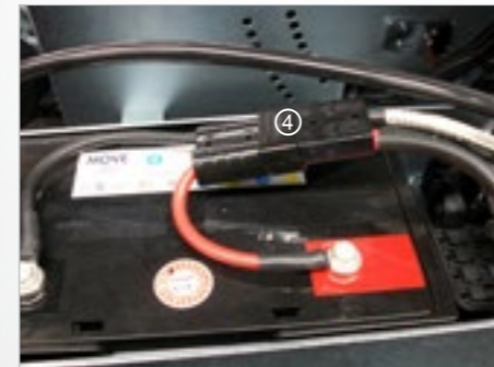
Fig. 54: Main Cable battery
