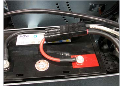
Fig. 47: Main cable battery
