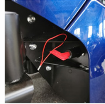
Fig. 95: Battery disconnect switch
