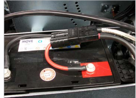
Fig. 39: Main cable battery
