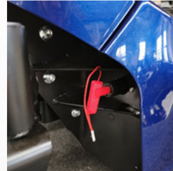
Fig. 96: Battery dicon. switch, inactive
